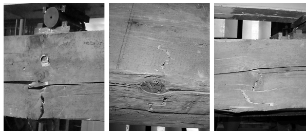
Fig. 6. Forms of beam destruction – from the left beams: BD6, BD5, BD2
